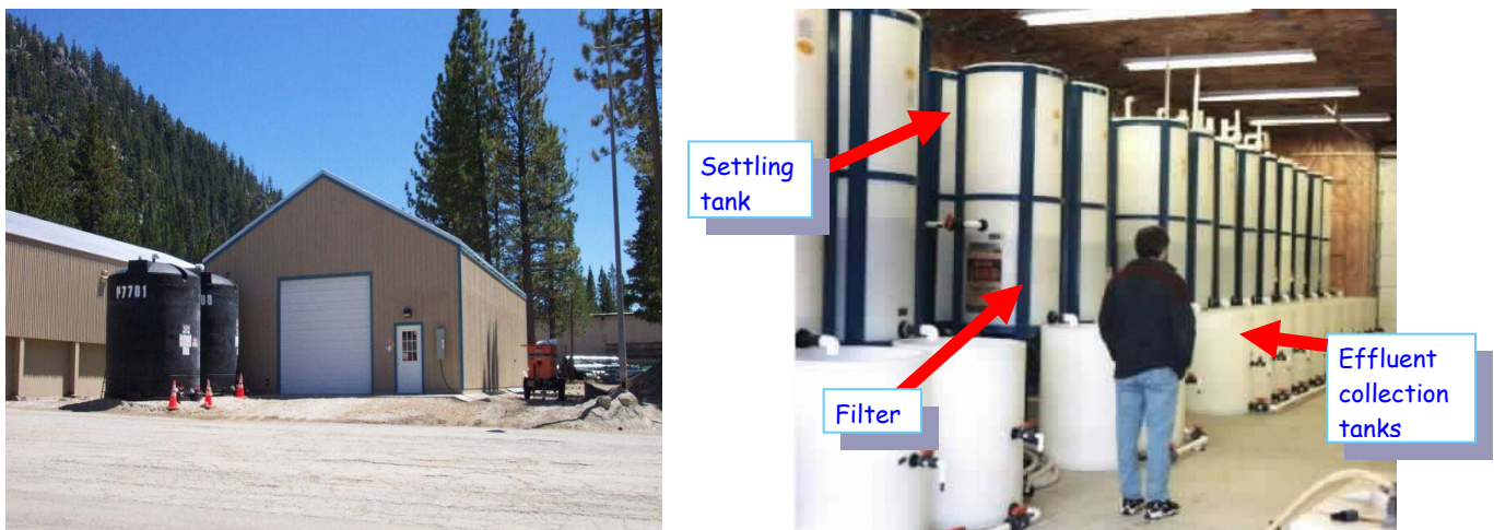
Figure 1 Photographs showing (a) pilot treatment building with storage tanks, and (b) sedimentation and filtration units
